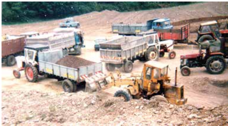
1980's: Work in progress for the Canovee GAA Pitch at Carrigadrohid. Pic Peter Scanlan
