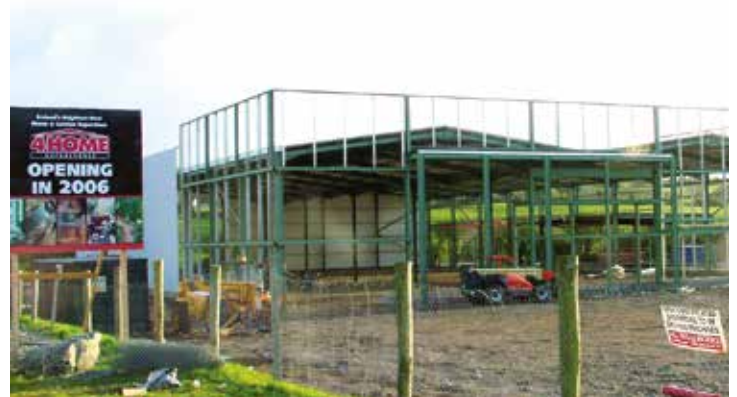
The 4HOME store in Macroom under construction in 2005. (Now the new Lidil Store). © Peter Scanlan
